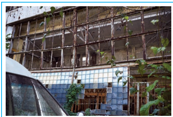
Building of V. Bakul Institute for Superhard Materials after missile attack, Kyiv
